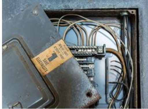
Figure 3: Electrical fire hazard. Source: Hassan, (1999)
